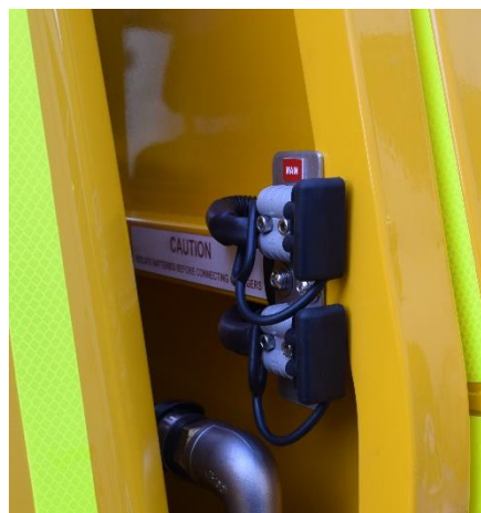
Figure 62: Battery Charger Connectors
