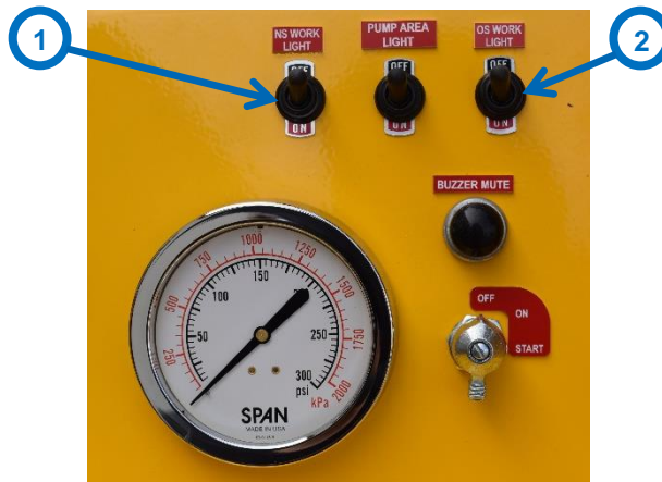
Figure 66: Lighting Controls - Pump Control Panel
