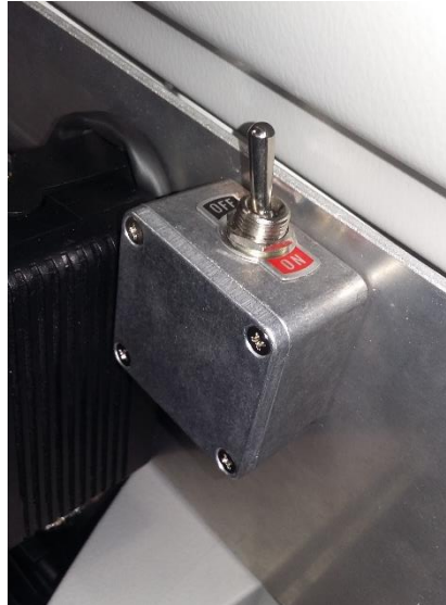
Figure 71: Water Level Indicator Isolation Switch
