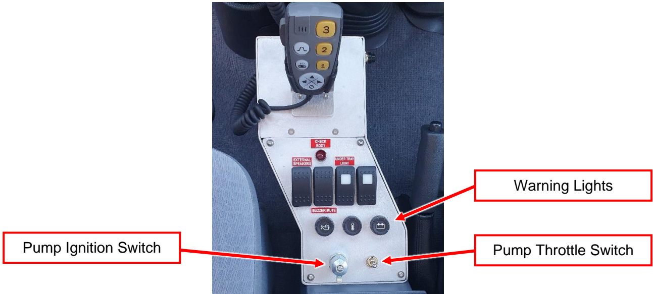
Figure 31: Pump Control Panel – Cab.
